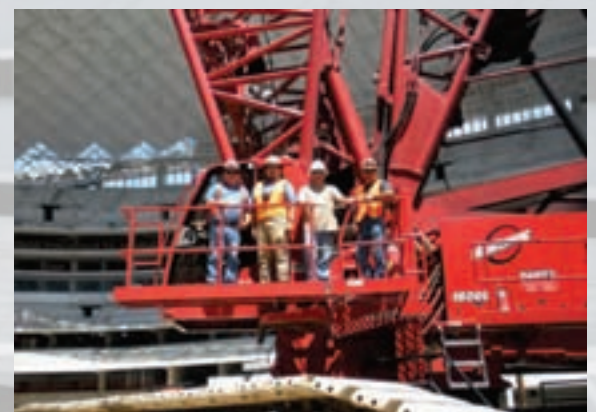
Local 178's Rodney Maxwell, 18,000 Manitowoc operator; Robert Teran, Local 178 business agent; Chris Hardy, 918 Link Belt operator and Assistant Safety Coordinator Cesar Jaquez for Derr Steel Erection at the new Cowboys Stadium.
